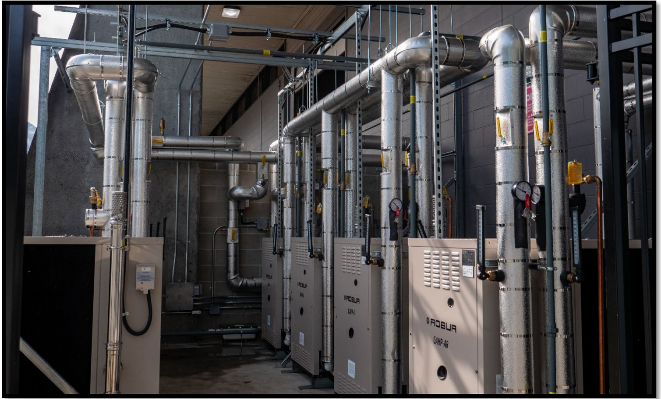
Figure 2 – Gas Absorption Heat Pumps installed at the UFV Trades and Technology Centre
